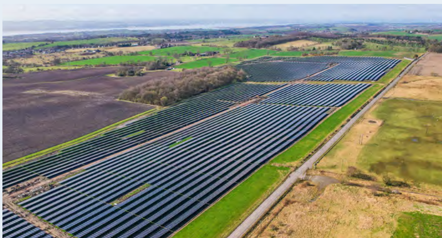
📍 Solar PV at Dunfermline
