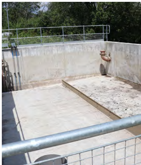
North Petherwin storm tank
