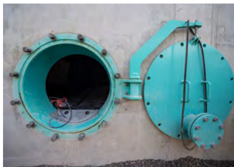
① Alderney Water Treatment Works, Bournemouth Water
