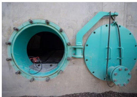
📍 Alderney Water Treatment Works, Bournemouth Water
