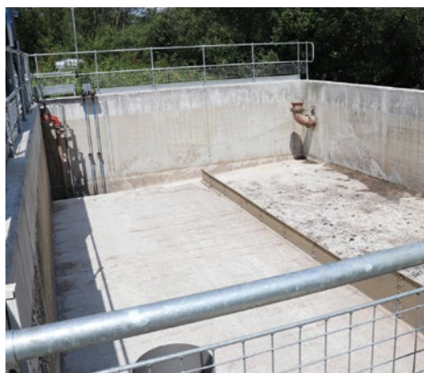
📍 North Petherwin storm tank
