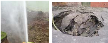
Scenes like this are what we want to avoid by replacing more and more water mains. At the moment, the funding available means they are expected to last 300 years!
